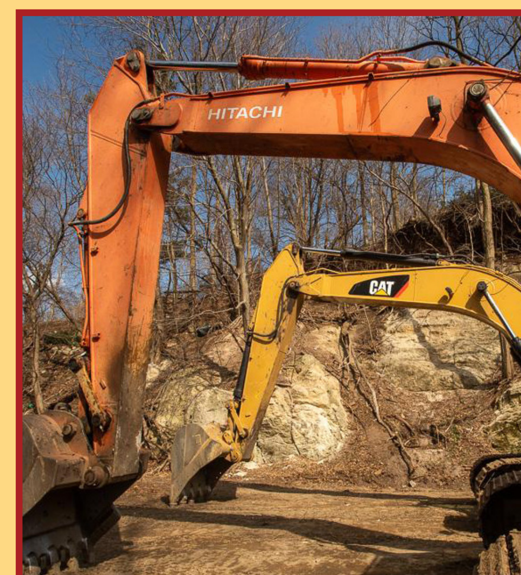
Backhoes on east side of quarry in early 2020. PHOTO COURTESY OF JIM METZGER
