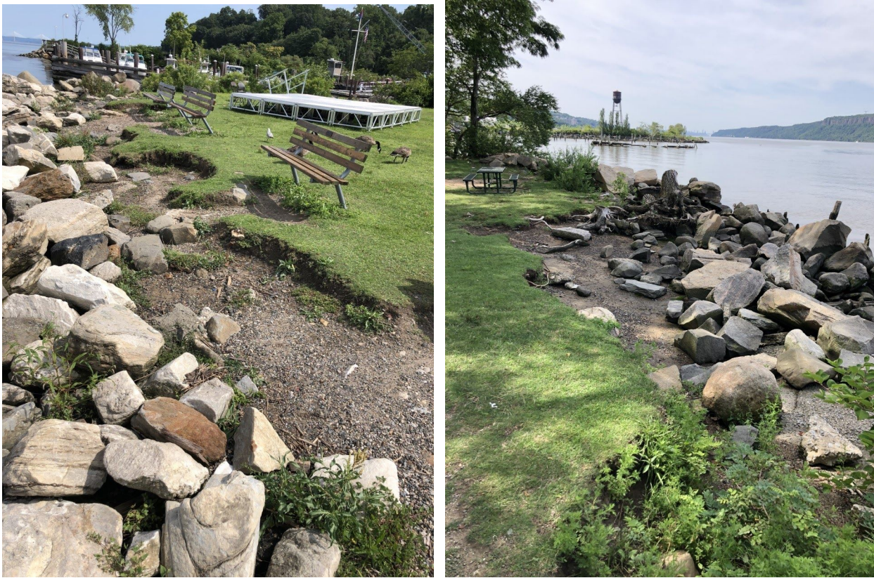
Appendix Figure 4: Erosion along the Hudson River shoreline at MacEachron Park.
