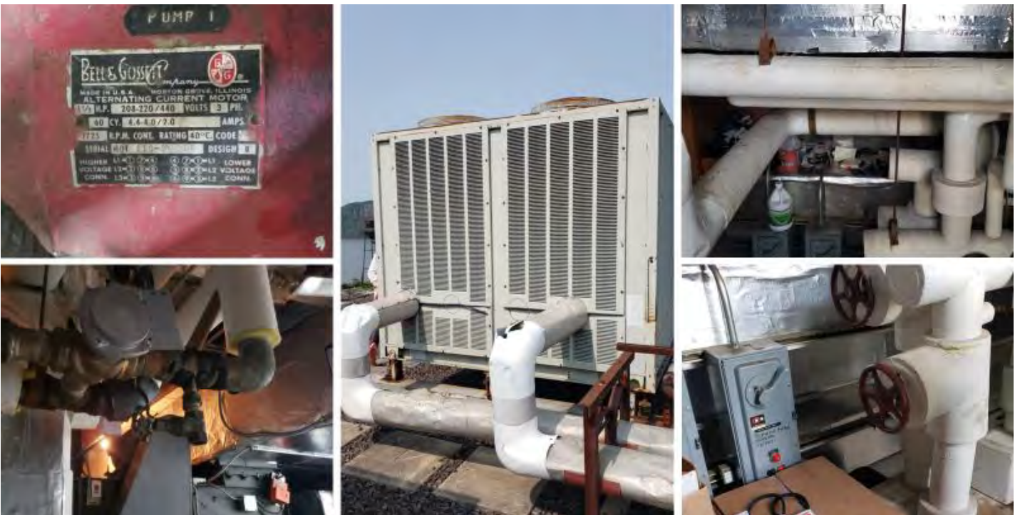
Figure 6. Cooling systems at the Village Hall and Library
