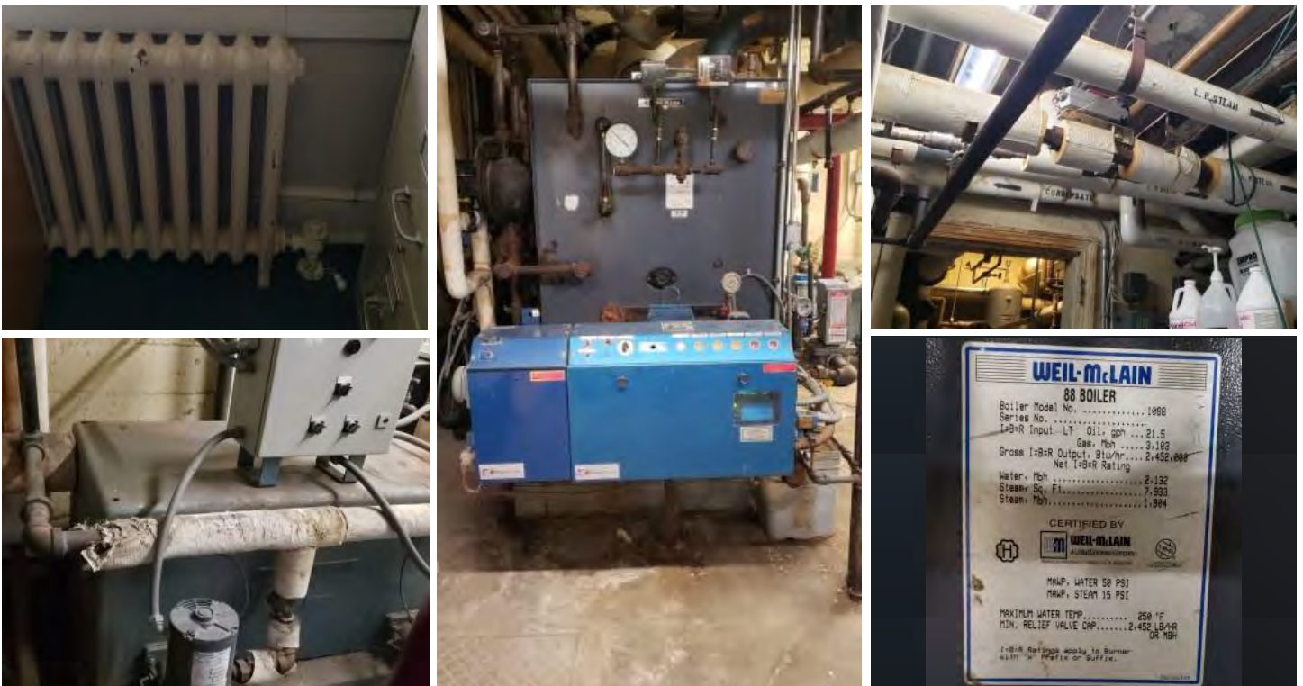
Figure 5. Heating systems at the Village Hall and Library
