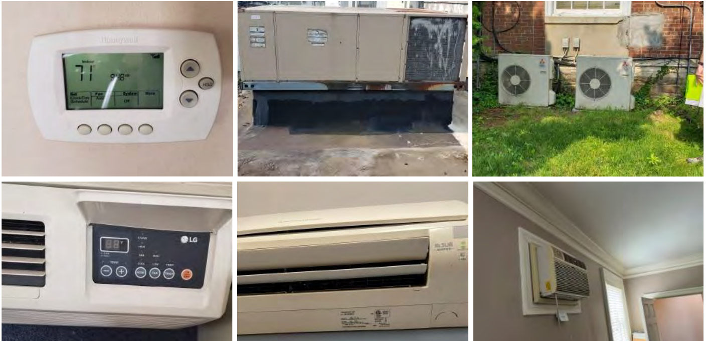
Figure 7. HVAC terminal systems at the Village Hall and Library
