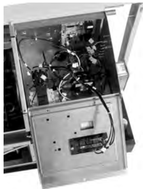
Figure 11. Hinged control box
